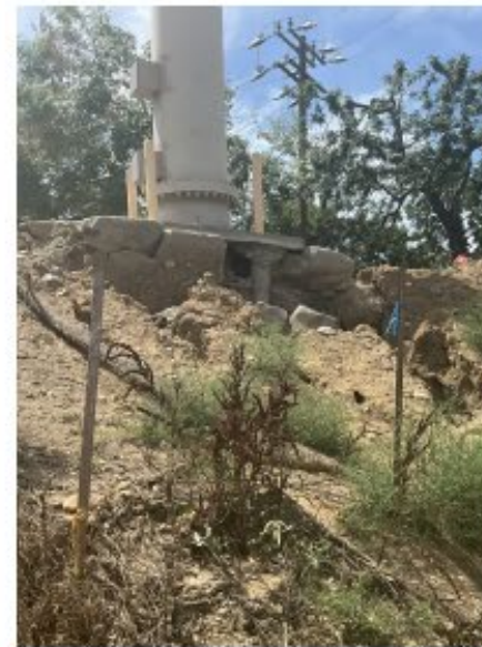
Shotcrete Void Below Concrete Slab
